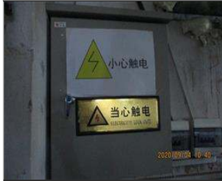
Photo of the inside of the main production hall Electronic protection.JPG
