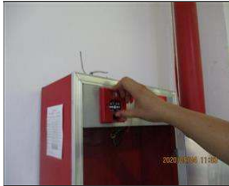
Photo of fire safety equipment Fire alarm test.JPG
