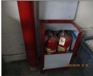
Photo of fire safety equipment Fire extinguishers.JPG
