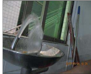
Photo of chemical storage room (if applicable) Eye wash facility.JPG
