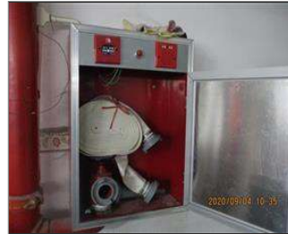
Photo of fire safety equipment Hydrant and fire alarm.JPG
