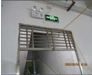
Photo of fire safety equipment Emergency light and safety exit sign.JPG
